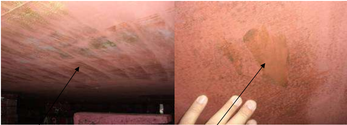
Slime layer remained due to lack of washing down.
